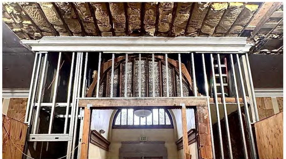
The University Branch retrofit includes a steel moment frame at the front entrance.
