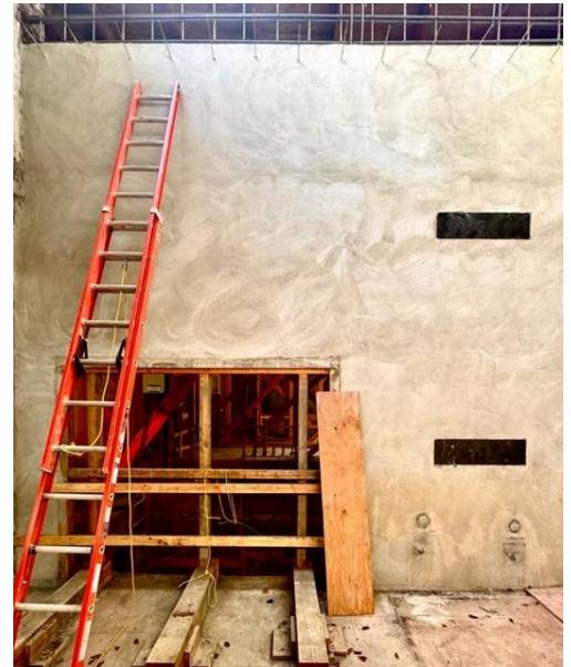
Reinforced concrete shear walls for future study rooms at the University Branch.
